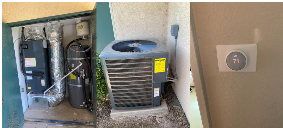
Figure 3. Pre-retrofit heat pump and heat pump water heater
